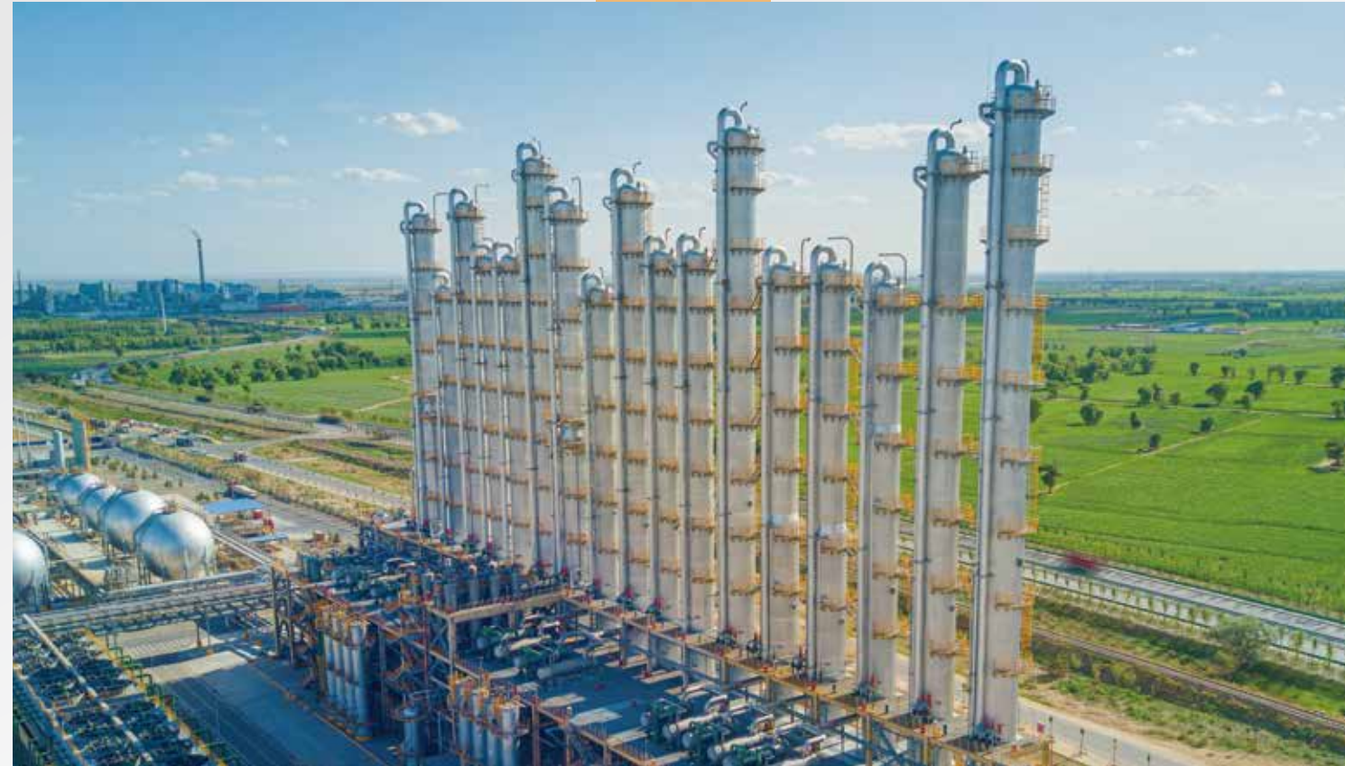
Tongwei Rectifying Tower Unit
